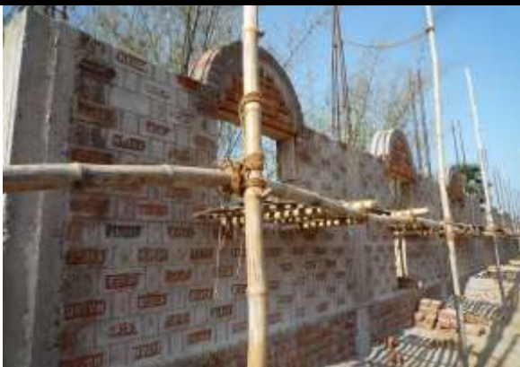
Arches not cement lintels
